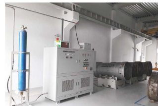
Refrigerant Outside Supply Equipment
