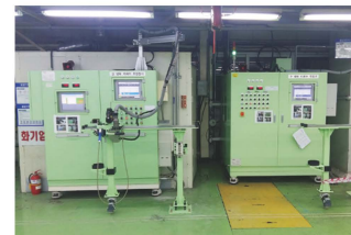
Repair Filling Equipment
