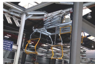
Over Head Conveyor System
