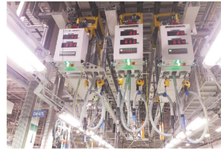
Refrigerant Charging Equipment
